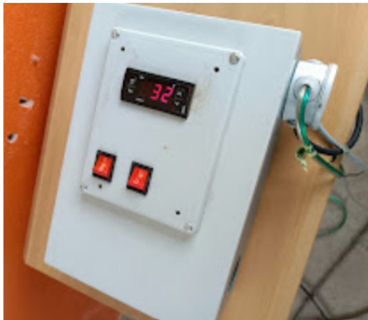
Figure 3. Control box of the setup
